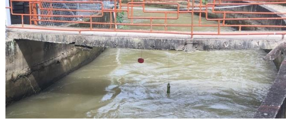
Level measure system. Usorrecio, Tolima-Colombia Image taken by the author on June 2018
