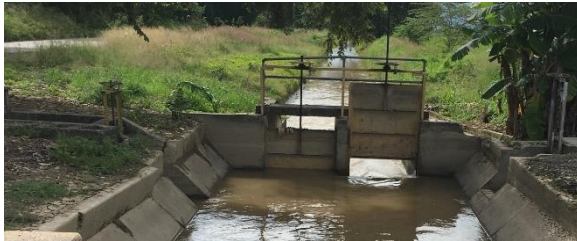
Discharge structure. Usorrecio. Tolima-Colombia Image taken by the author on June 2018
